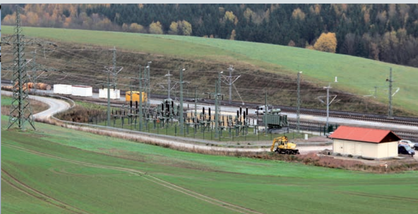
Traction substation on the new Erfurt–Leipzig/Halle line in the Saubachtal in the Burgenlandkreis district
