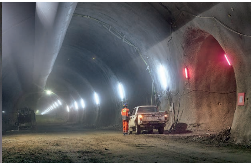
Rescue tunnels branching from the main tunnel, Baumleite Tunnel 2010, new line Ebensfeld–Erfurt (VDE 8.1)
