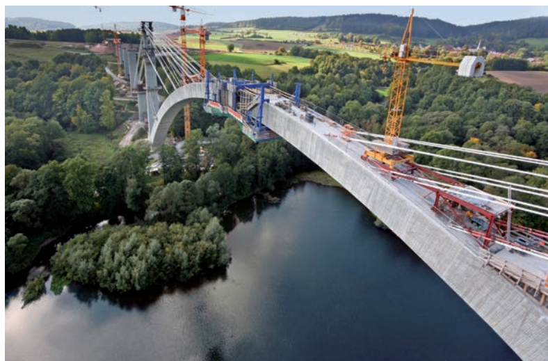
Arched bridges in the Thuringian Forest with record span widths to conserve the valley floor, Froschgrundsee Viaduct 2009, new line Ebensfeld-Erfurt (VDE 8.1)
