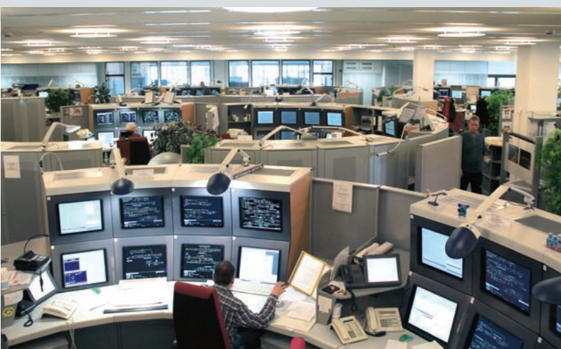
Electronic signalling technology, control centre in Leipzig 2013
